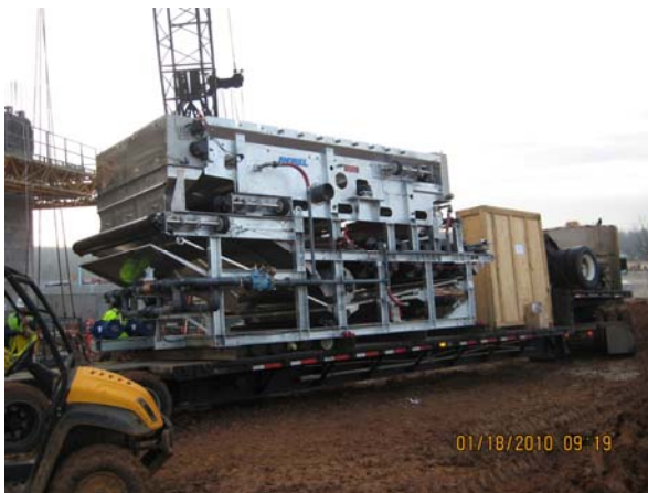
Belt Filter Press delivered on truck
