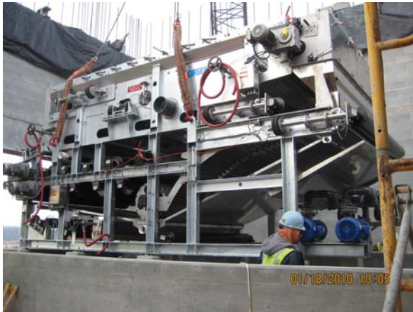
Belt Filter Press in Sludge Process Bldg.
