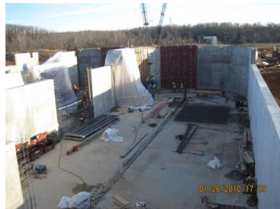
South end of Process Train 41
