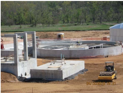
Clarifier 62 and Return Sludge Pump Sta.
