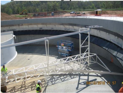
Current baffles in Clarifier 62
