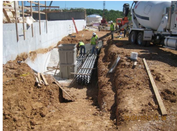
Electrical duct bank at HH-04-2
