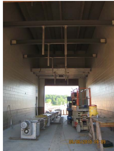
Conveyor supports in Sludge Process Bldg. truck bay
