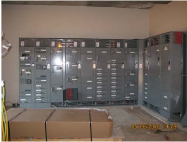
Sludge Process Bldg. electric room
