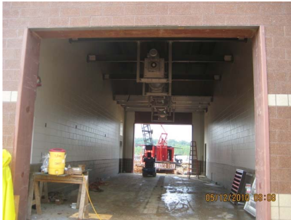
Conveyor in Sludge Process Bldg. truck bay
