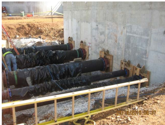
Piping between Return Sludge Pump Sta. & Valve vault
