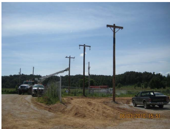
Power poles for power feed into plant
