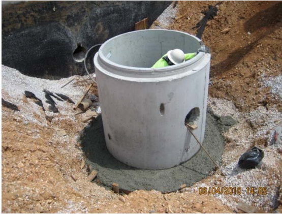
Oxygen Injection manhole
