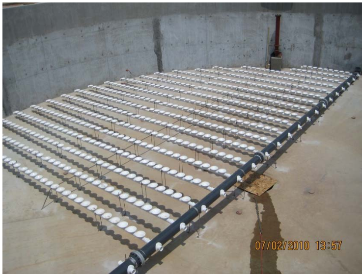
Diffusers in Sludge Storage Basin
