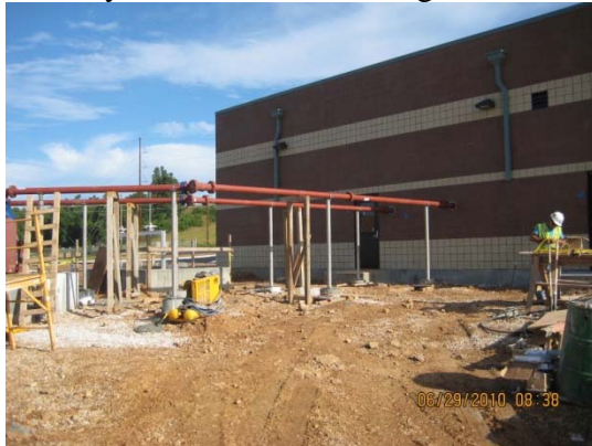
Grit piping between Grit Chamber and Screen Bldg
