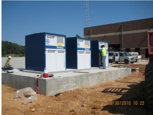
Blowers at Sludge Storage Basin
