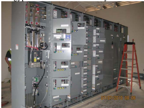
Motor Control Center in Control Bldg. #1
