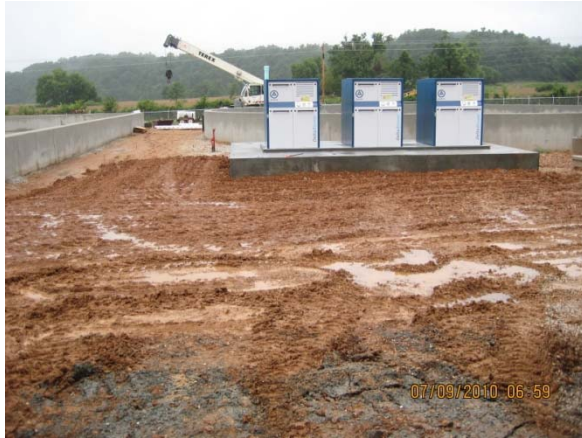
Muddy conditions at Sludge Blowers
