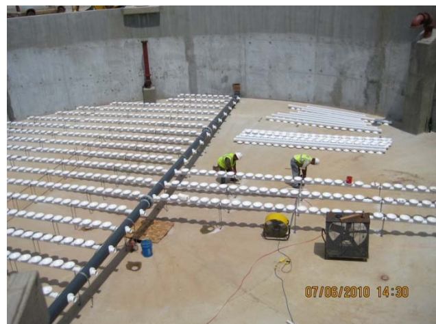
Photo 2: Sludge Storage Basin Diffuser Piping.
