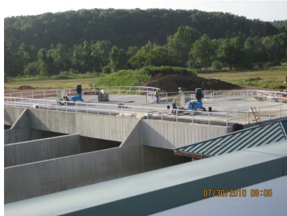
Process Train south deck
