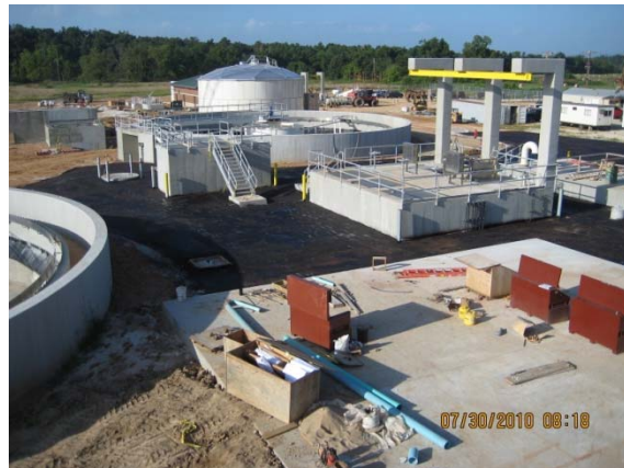
Return Sludge Pump Station area
