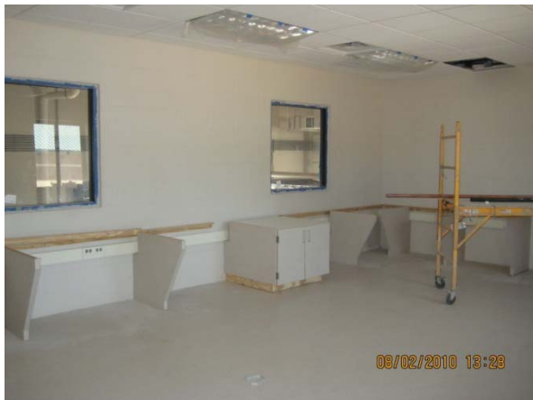
Sludge Process Bldg. control room
