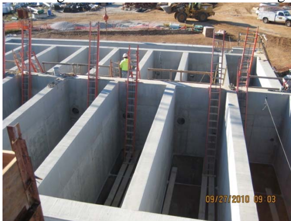
Filter bldg. cells
