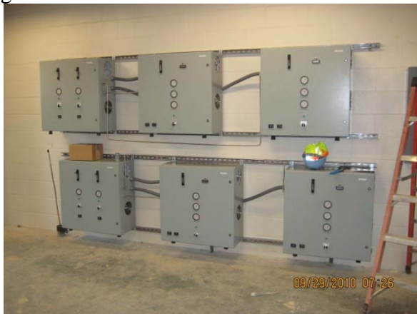
Oxygen generation cabinets
