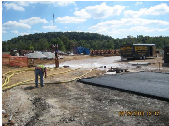
Pumping test of fire pumps
