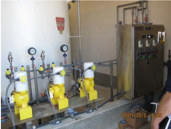
Alum Pumping system
