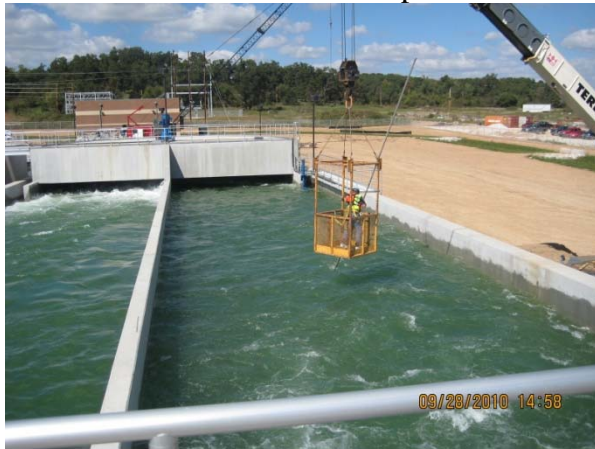
Velocity testing in Process Train
